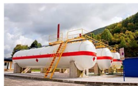
Tank Flow Monitoring
